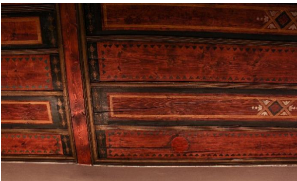
Figure 1: Detail of the wooden ceiling decorated with oil paintings on the second floor (picture taken in 2016). Cracks are visible along the tangential direction of wood panels.
