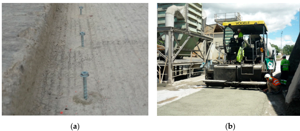
Figure 10. Screw anchors in the milled surface (a). Asphalt paver extending the concrete (b).
