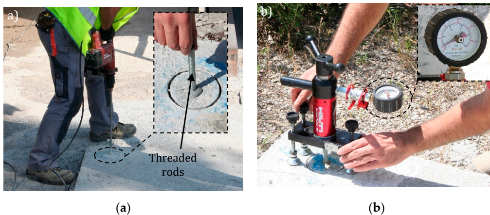
Figure 7. Pull-off test: drilling and placing of threaded rods (a) and anchor tester (b).
