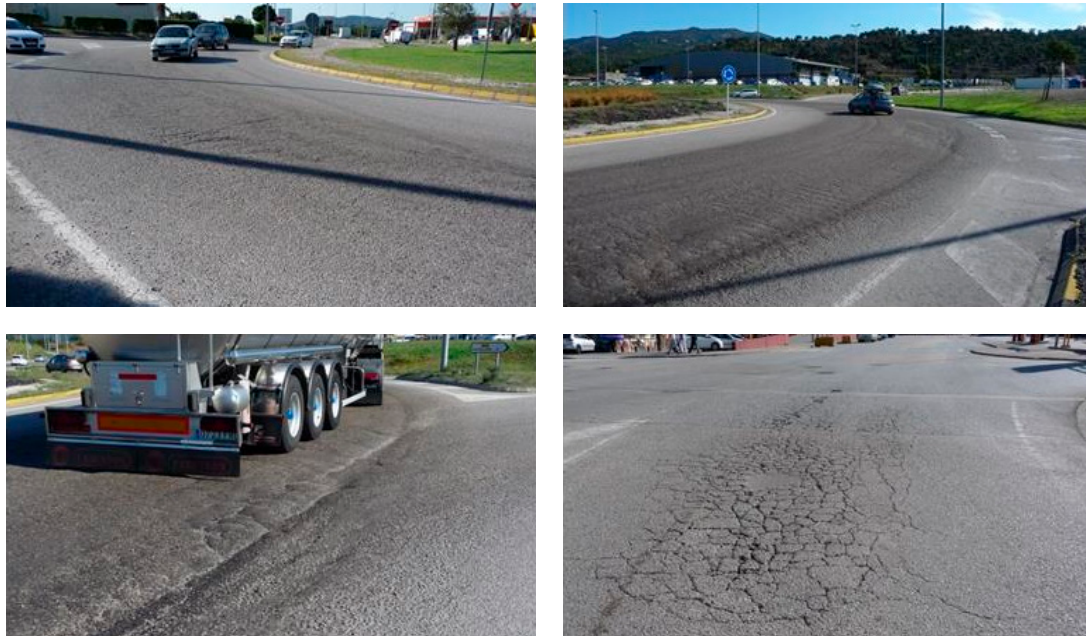
Figure 12. Previous pavement condition of the roundabouts.
