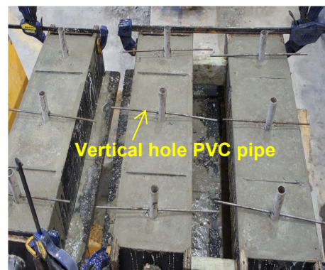
Figure 8: Vertical holes connecting with the sleeved encapsulation hold for sleeved bolt encapsulation
