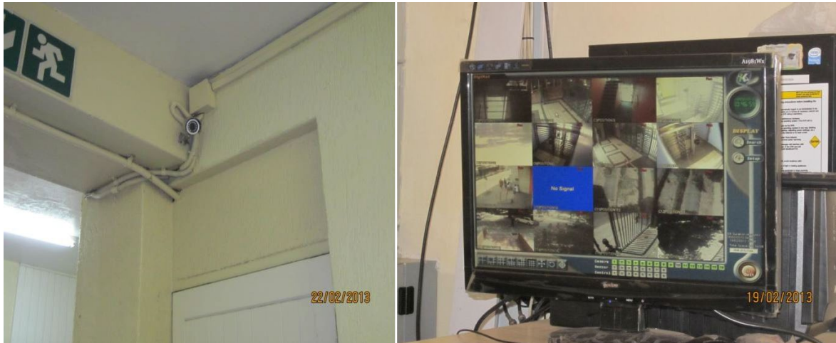
Image 3: CCTV surveillance equipment inside social housing buildings, Hillbrow (photographs by the author)
