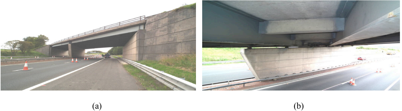
Figure 1. The Stirlingshire link motorway bridge [18]: (a) looking downlink on M9; (b) detail view of steelwork typical.
