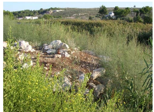
Torrente Macinino. One year after the works of renaturation of the river morphology.
