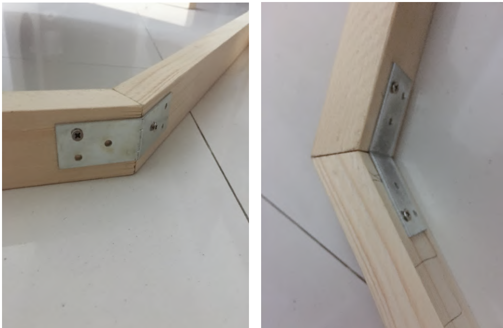
Figure 4.16 Fixing eight sections of the wooden frame by using angle steels and screws
