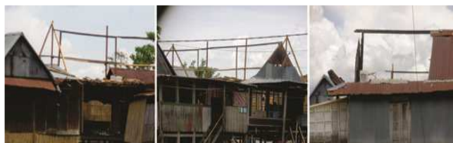
Fig. 4. Roof sheet flew with the wind
