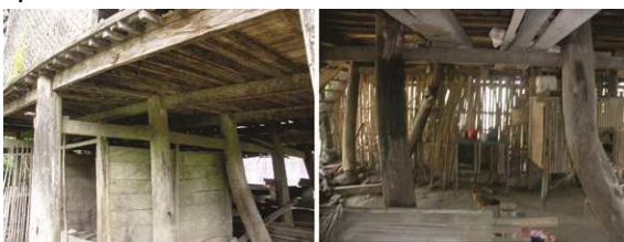
Fig. 1. Bent column in center position
