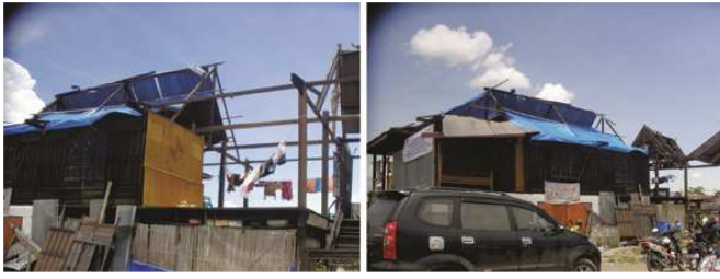
Fig. 6. The wind destroyed part of the wall
