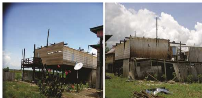
Fig. 5. The roof structure destroyed by the wind
