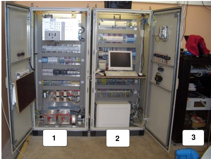
Figure 2.4.: ATOM control electronics. Some main components: cabinet 1, upper part : manual control panel used for on-site control without any computer involved; bottom : transformers for the telescope servodrives; cabinet 2, 2nd panel from above : main PLC of control system; bottom : telescope control PC attel (relocated to cabinet 3 in the meantime). cabinet 3 : computer for instrument control, network and telephone access for ATOM building.
