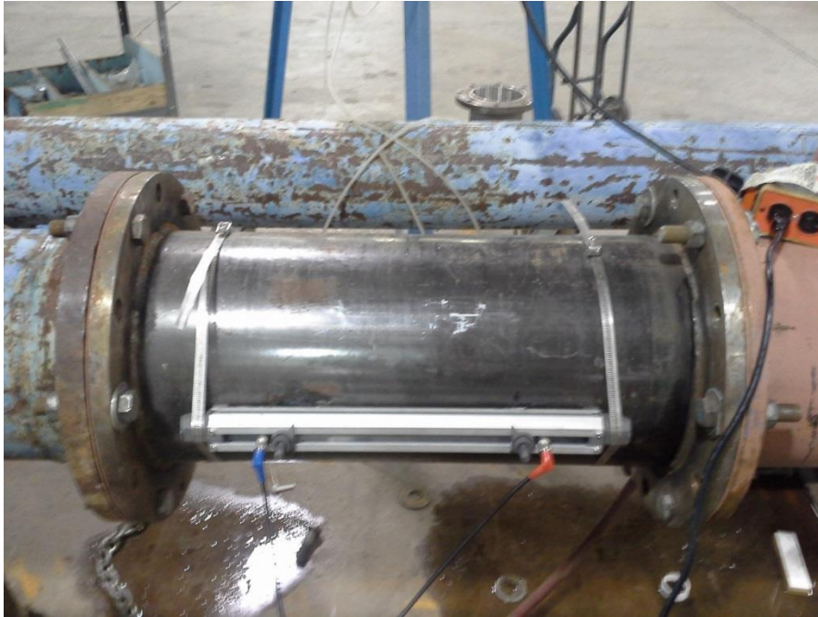
Fig. 16. Ultrasonic flow meter installation.
