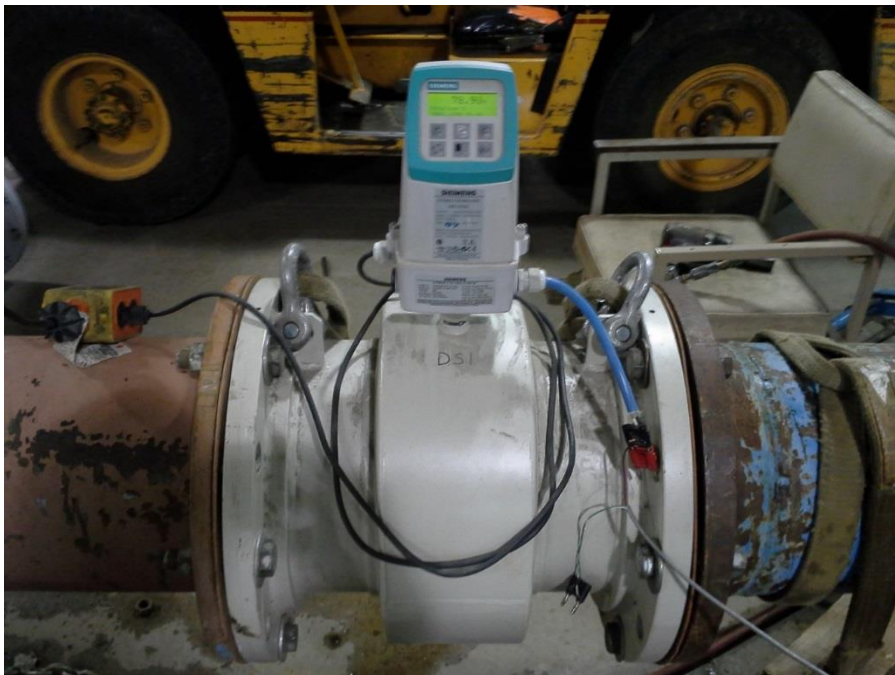
Fig. 14. Magnetic flow meter installation.
