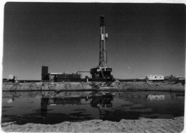
Figure 1. A typical oil well drilling rig and waste pond. Drilling fluids (muds) are needed to cool the bit, seal porous geologic strata, and float rock cuttings out of the bore hole. The mud tanks, left of the rig, appear in the photo as the long flat tanks. Barite for making new mud is in the tall blue hopper at the left edge of the rig. Sacked mud ingredients (bentonite, sodium hydroxide, lignite, and others) are housed in the shed (white) just between the barite hopper and the mud tanks.
