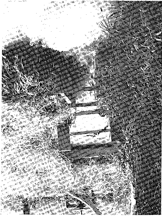
Fig. 34. Parshall flume located below structure 14HW.
