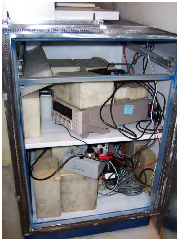
FIG. 3.7. Metal electronics enclosure located below the RIC chamber. Additional polyblocks were placed so as to provide additional radiation shielding (left).
