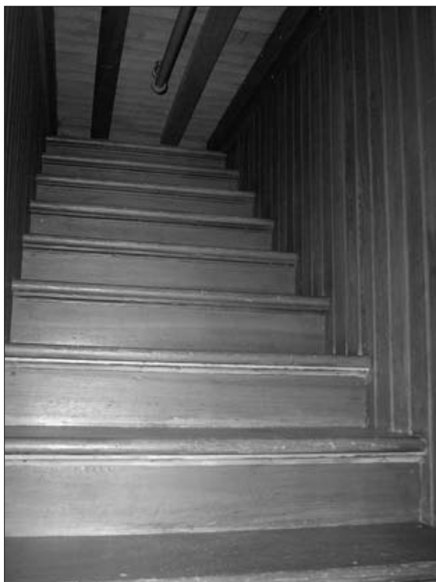
FIGURE 3: The oft-photographed staircase leading to nowhere demonstrates the mansion's dysfunctional qualities, Winchester Mystery House. San Jose, California. (Photo by Jeannie Banks Thomas)
