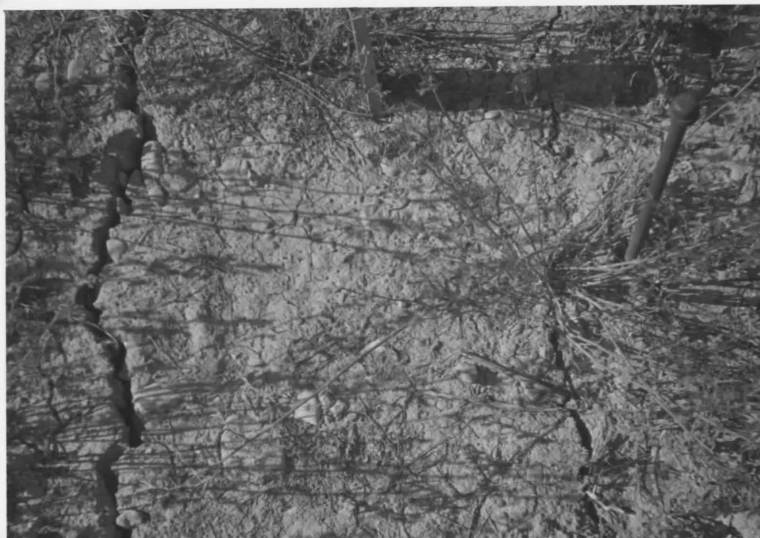
Figure 24. Shrinkage cracks in the clay soil
