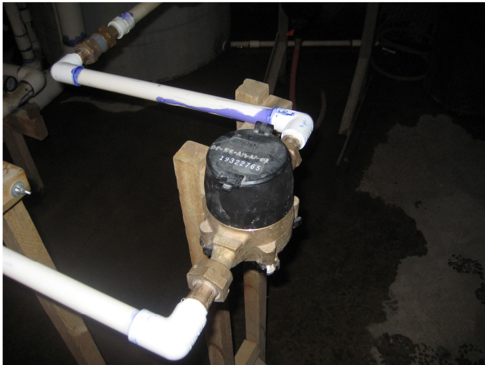
Figure 6. 90 degree elbow upstream of meter
