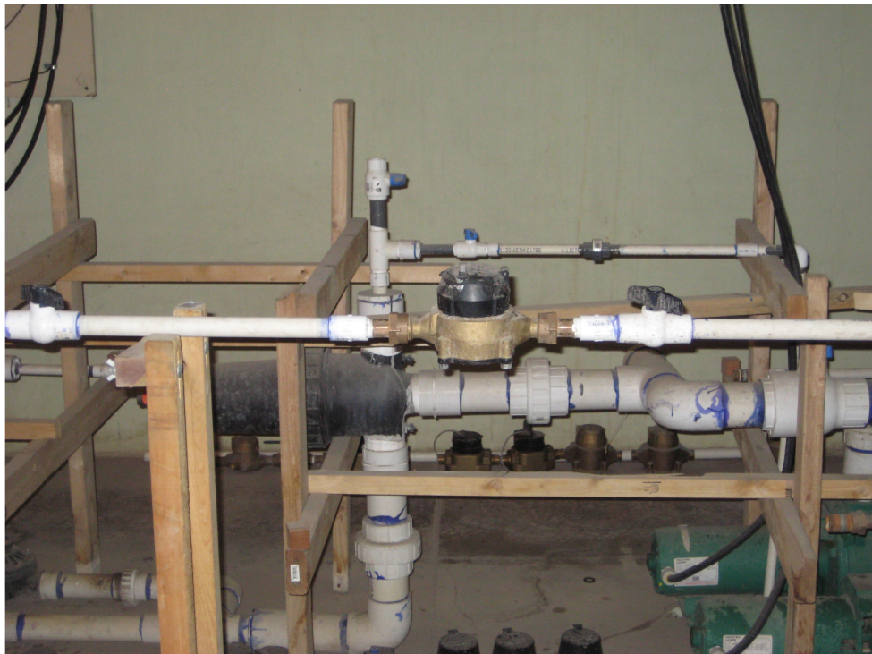
Figure 10. Partially open valve
