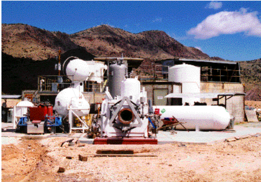
Figure 3. 80,000-lb. Thrust Engine Test Stand at the Energetic Materials Research Test Center (EMRTC) Rocket Test Site at Socorro, NM. The facility will be used to test the Microcosm 5,000-lb., 20,000-lb., 40,000-lb., and 80,000-lb. thrust engines.
