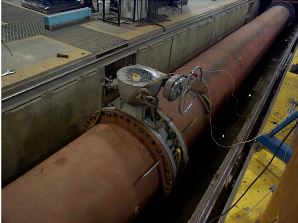
Fig. 2.1: Example of a butterfly valve installed in a pipeline at the UWRL.
