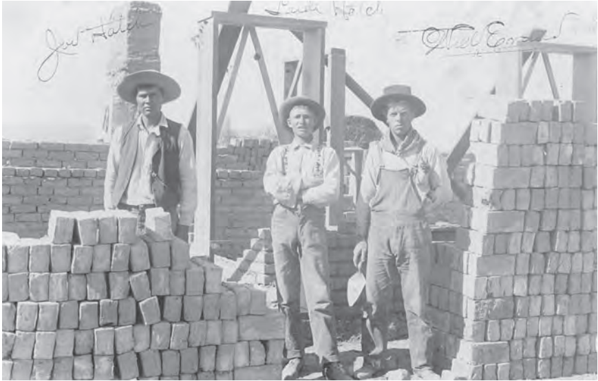
Joe Hatch, Sr., Lude Kirk Hatch, and Will Evans building James “Grandpa” Pipkin, Jr.’s house, June 1897 in Fruitland, New Mexico. This was shortly before Evans’s initial trading experience at Sanostee.
