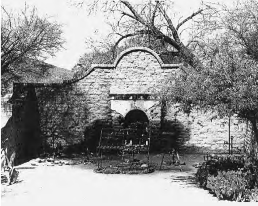
El Tiradito from the east, May, 1992. The central object in front of the wall is a wrought iron candle rack; other metal candle holders are visible to either side. The discoloration of the central part of the wall is from candle smoke; the dark stain on the ground is from candle grease. Photograph by James Griffith.
