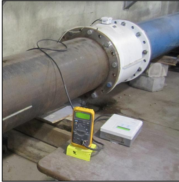
Fig. 13. Multi-meter attached to mag-meter.
