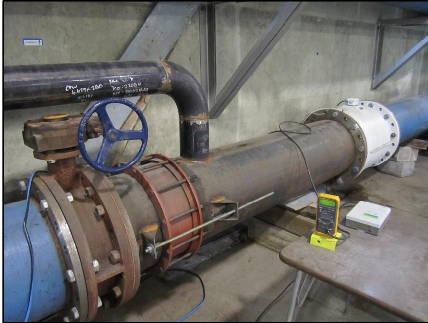
Fig. 7. 20-inch (50.8 cm) supply line with mag-meters.
