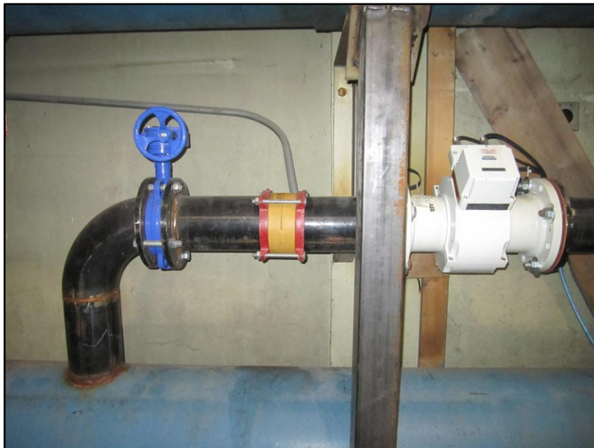
Fig. 8. 6-inch (15.2 cm) supply line with mag-meters.
