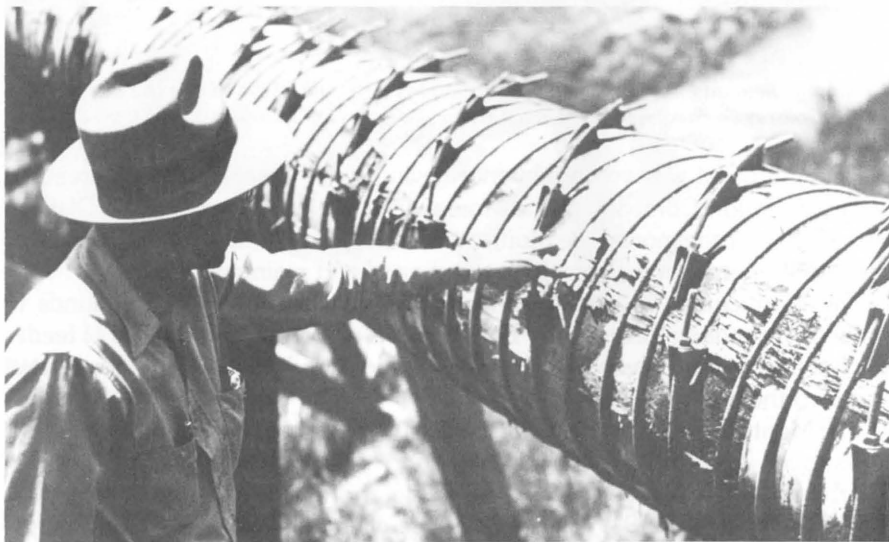
Repairs associated with wooden siphons like this one at Alkali Draw proved to be a continual financial drain on the troubled irrigation system. (Dolores Archeological Program Records, Dolores, Colorado)
