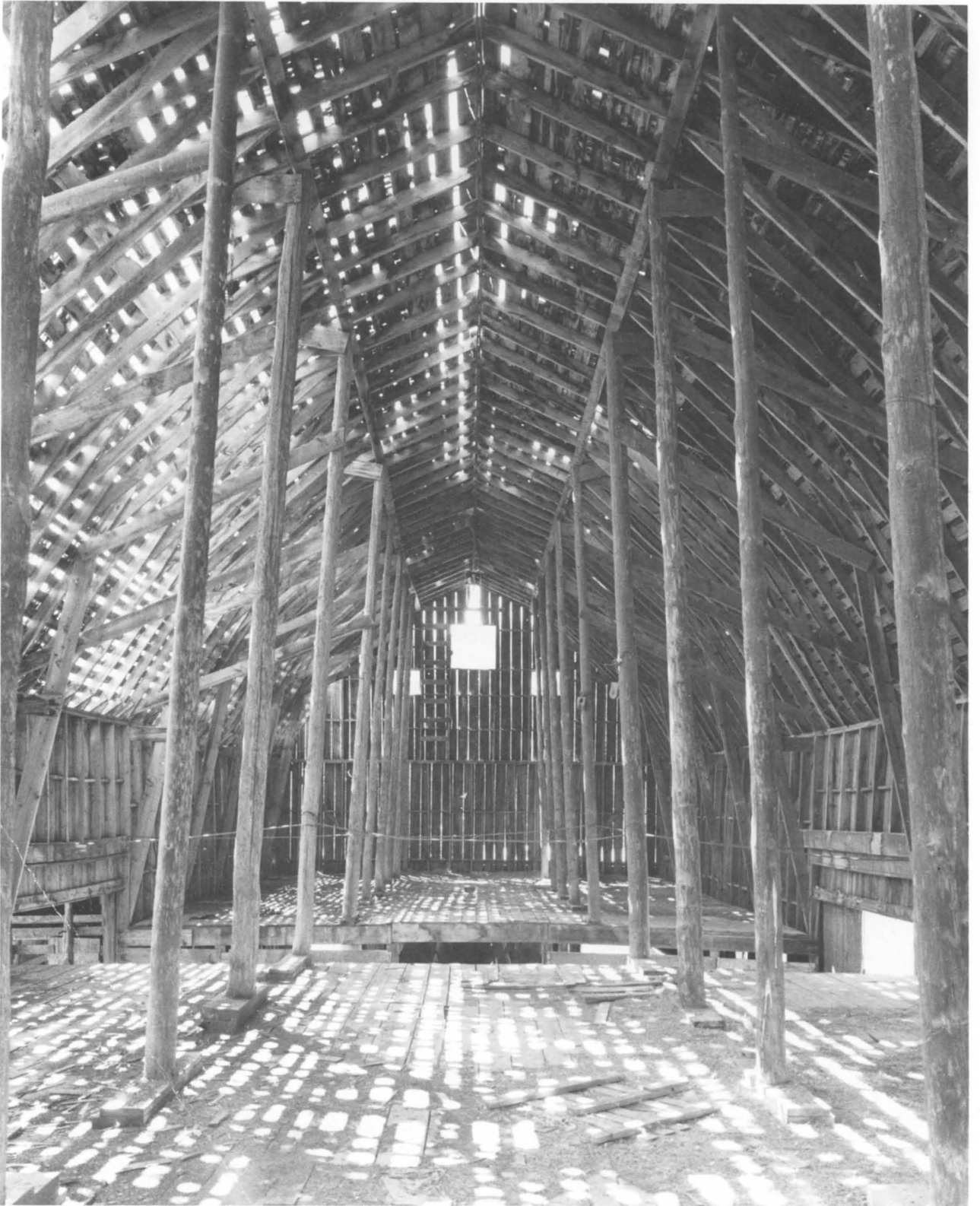
Although time has taken its toll, the interior loft of the barn remains impressive. (Jet Lowe, HAER)
