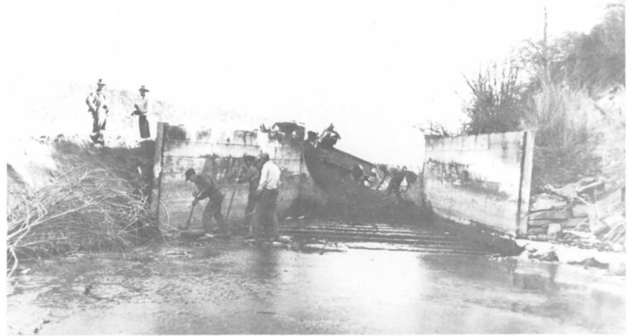
In order to reduce maintenance costs, the Morton Flume was replaced by a metal and concrete ditch which carried twice the capacity of the old flume. (Dolores Archeological Program Records, Dolores, Colorado)
