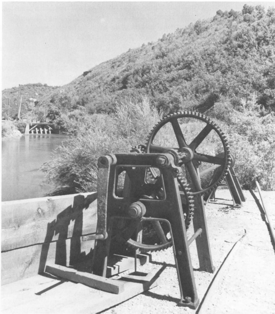
This headgate mechanism controlled the intake to the tunnel, providing water to Montezuma Valley ranchers and farmers. (Jet Lowe, HAER)
