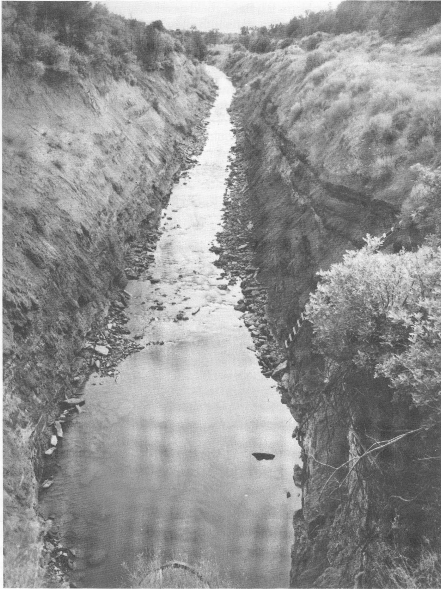
In November of 1885, hardy workers, including nearby ranchers and farmers who would later benefit from the irrigation system, began drilling, blasting and excavating the 5,400 foot Montezuma Valley Water Supply Company Tunnel. The outlet of the tunnel, shown here, was later reinforced in the winter of 1963-64 with steel arches. Sleeping Ute Mountain can be seen in the distance. (Jet Lowe, HAER)
