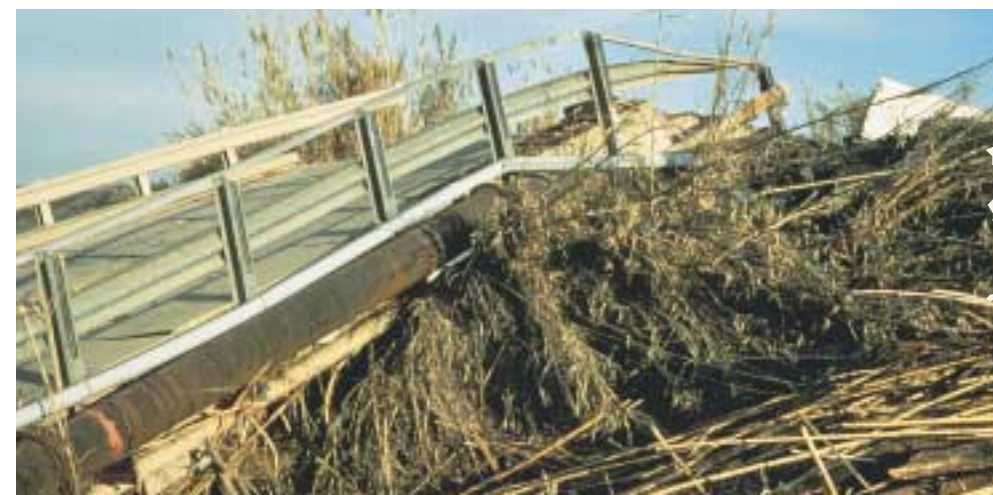
Giant reed clogs streams and rivers, sometimes threatening structures like this bridge. Photo courtesy of Tom Dudley.
