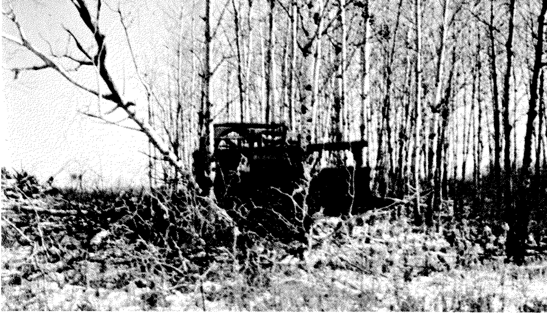
During the last few years, the Minnesota Division of Game has contracted for clearing substantial acreages of aspen land to convert them to desirable deer habitat. Shearing with a bulldozer was one of the methods used. Areas selected were impractical to log commercially.
