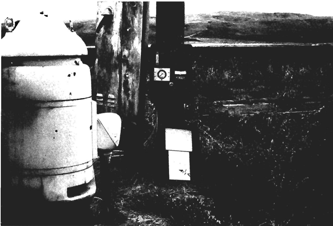
Figure 4. Low cost monitor unit.
