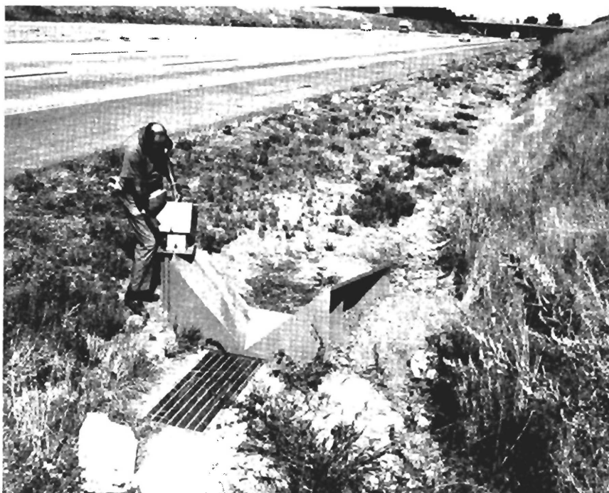
Figure 4. A view of the Layton site looking up the drainage channel—the paved portion and the cut slopes both drain toward the center and through the measuring flume.
