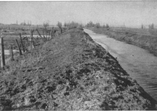
Fig. 1. A typical high irrigation canal, Lewiston area, that contributes to water logging soils
