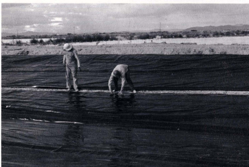
Figure 4. These strips of 10 mil. polyethylene film canal lining were seamed on the job. The strips were lapped 1 foot and sealed with mastic tape. After seaming, the earth cover was placed and spread.
