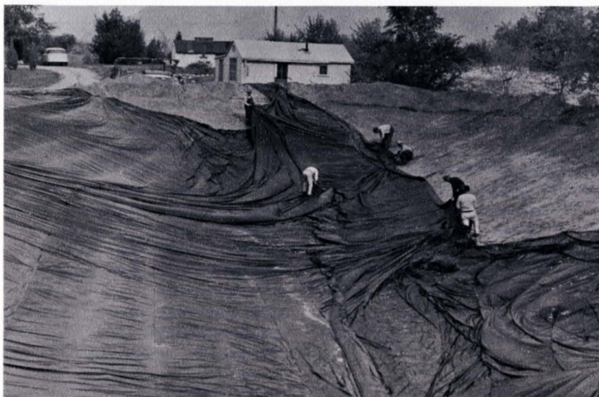
Figure 3. Parks Reservoir near Granite is lined with vinyl. Here, the film is being spread prior to placing the earth cover. The reservoir provides overnight storage of irrigation water.
