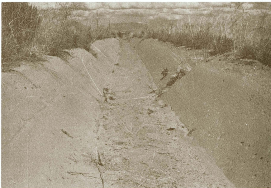
Figure 8. Condition of standard soil-cement lining with cement content of 14 percent on September 24, 1967—11 years after installation.
