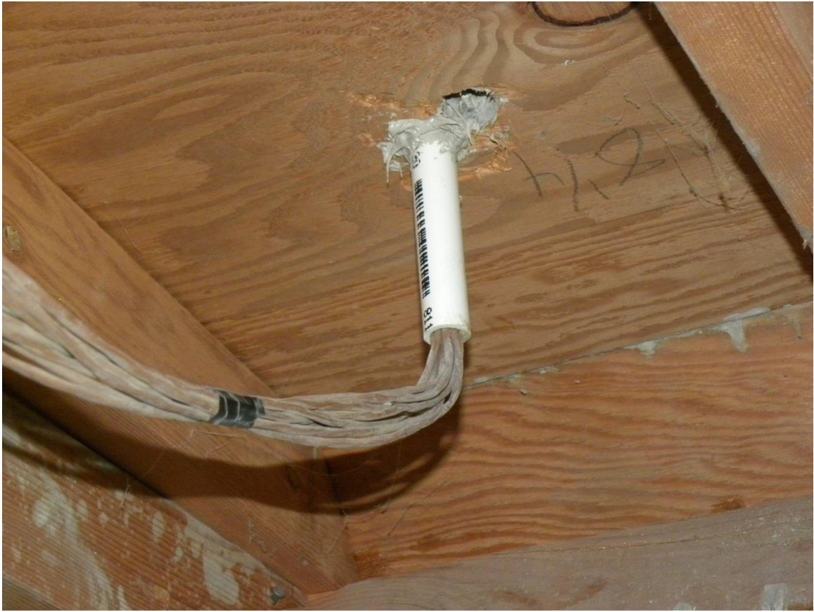
Figure 23 – Deck Thermocouples installed in the California Bridge.
