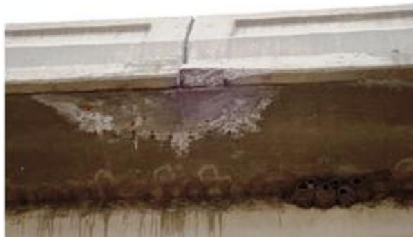
Figure 32 - Cracking at parapets on the Utah Bridge.
