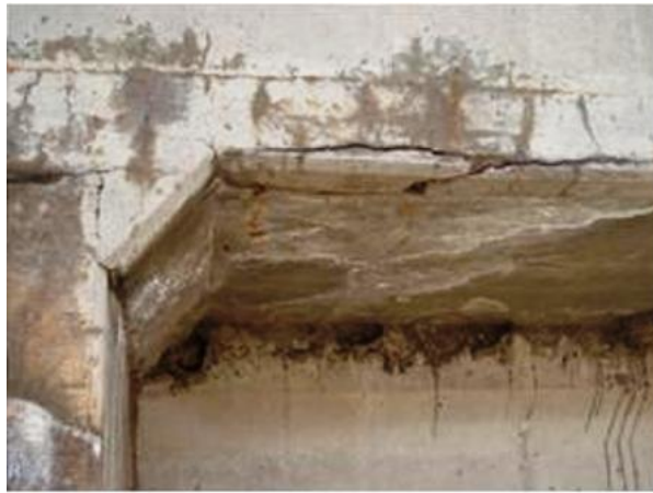
Figure 31 - Cracking at the abutment on the Utah Bridge.
