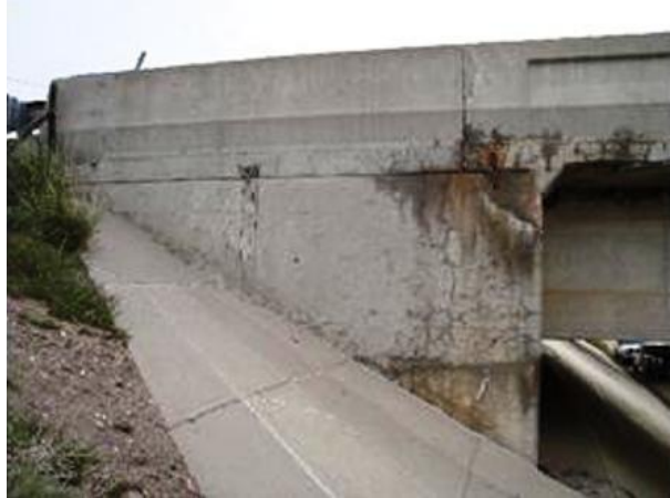
Figure 30- Cracking at the abutment on the Utah Bridge.
