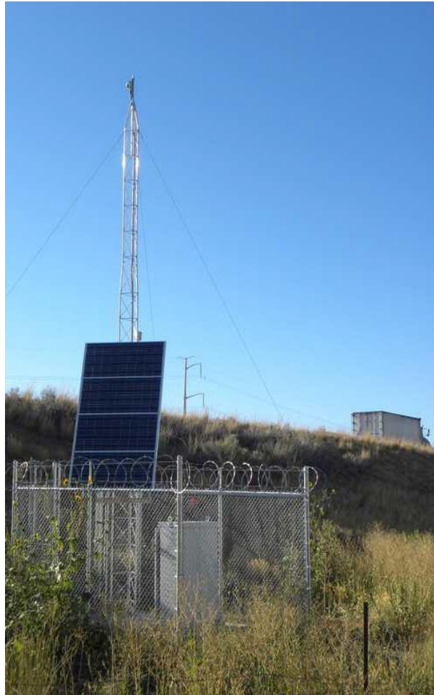
Figure 27 – Weather Station installed near the Utah Bridge.
