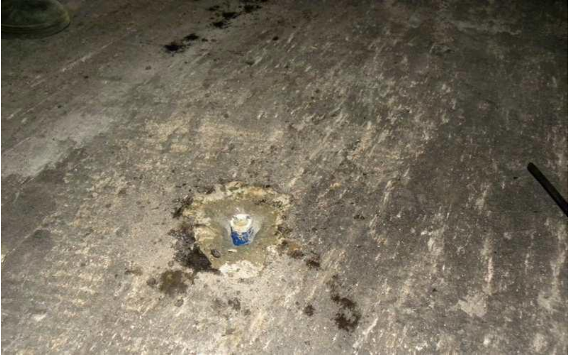
Figure 26 – Deck thermocouples installed in the Utah Bridge.
