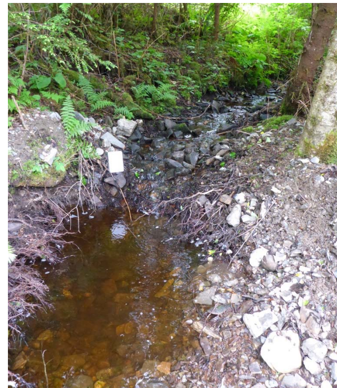
450 mm headcut moving upstream of embedded nonfilled pipe
