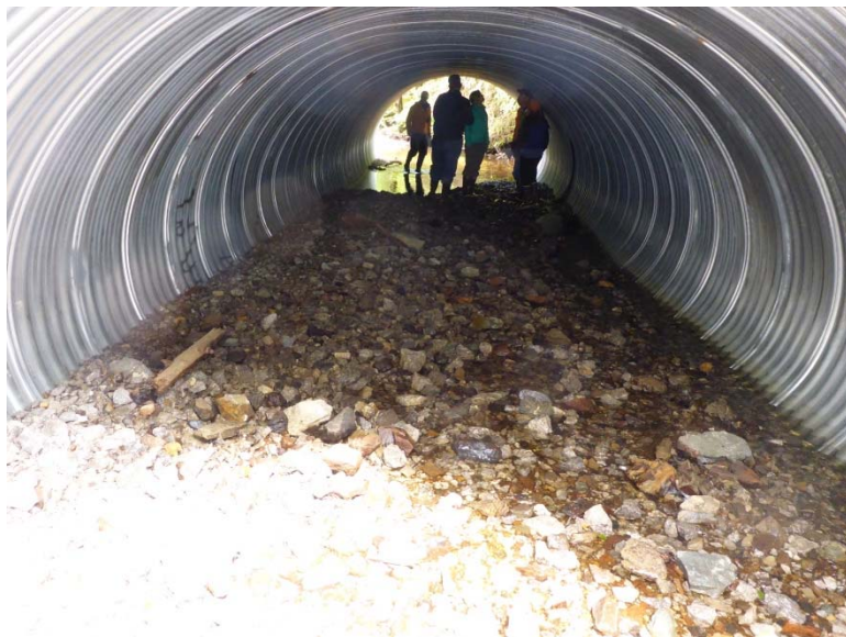
Self filled AOP structure Tongass NF, Alaska
