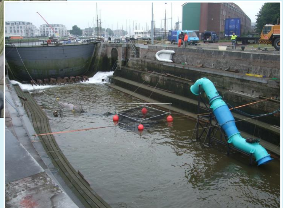
Pump and test rig
