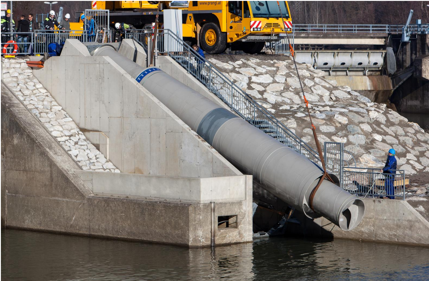
Fish screw at the Mur (Sulm) river
