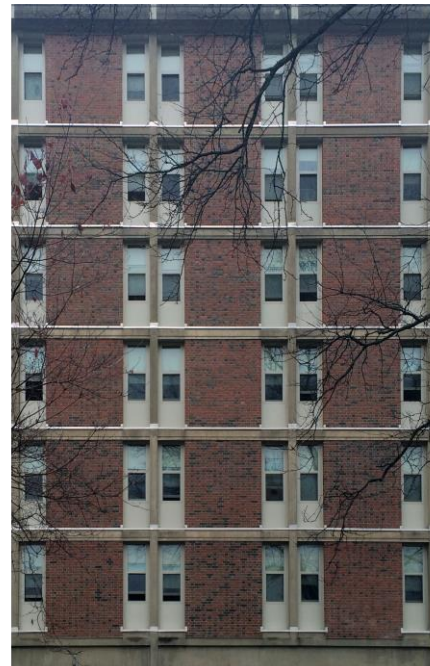
Figure 2: Thermal bridges with exposed concrete.
