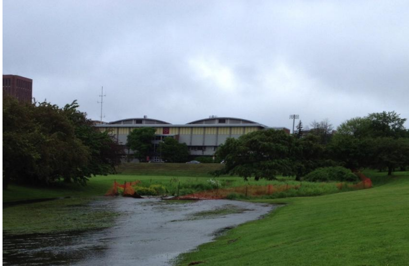
Figure 3.7: View looking east of a flowing stream and orange snow fence collapsing around the outlet pipe (photo credit: Nathan Frazee).
