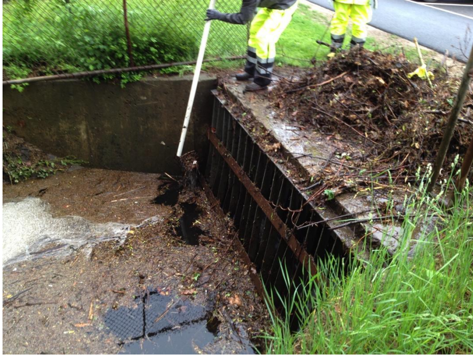
Figure 3.5: UMass Physical Plant teams work to clean out debris and sediment blocking the inlet drain at the Visitor’s Center parking lot (photo credit: Nathan Frazee).
