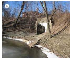
4. Cinched outflow pipe draining into restful spot by the River.
