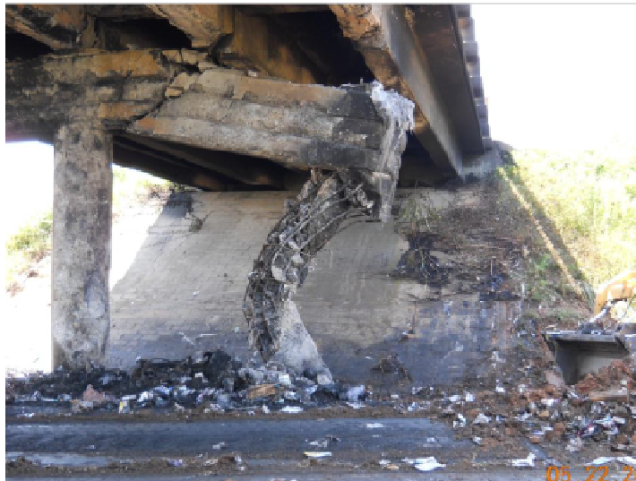
Figure 1.2. Damage caused by the tractor-trailer collision with the SC Highway 150 bridge over I-85 (Smoke 2012)
