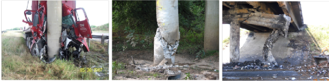
(a) (Buth et al. 2010) (b) (Buth et al. 2010) (c) (Smoke et al. 2012) Figure 6.40. Examples for (a) minor, (b) major, and (c) extensive damage states
