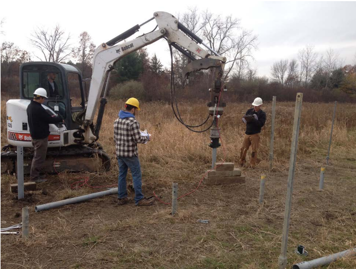
Figure 4.5 Torque Monitoring During Helical Pile Installation at UMass-DOE Site Using Bobcat 435 and Large Eskridge Hydraulic Head.
