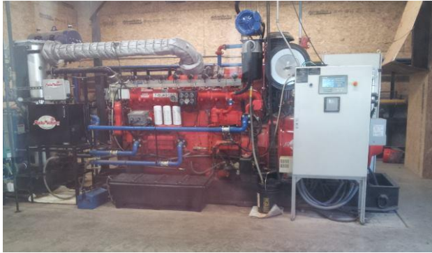
Picture 3: Barstow Farm Digester “cogeneration” Engine produces enough electricity to power 250 homes continuously
