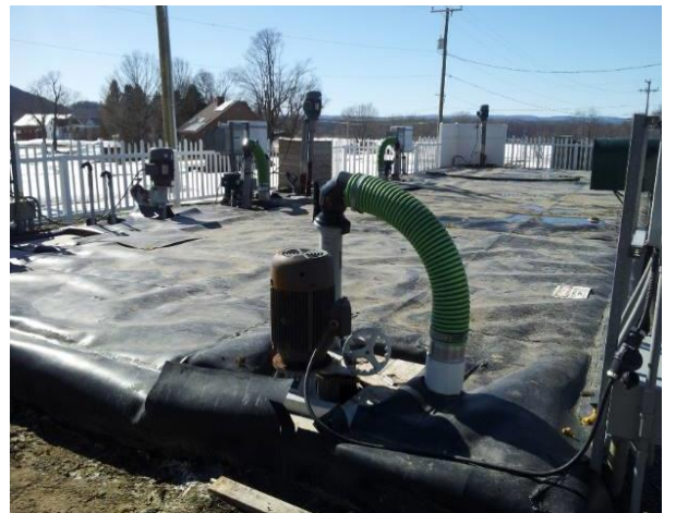
Picture 2: Separated Source Organic Waste Tank
