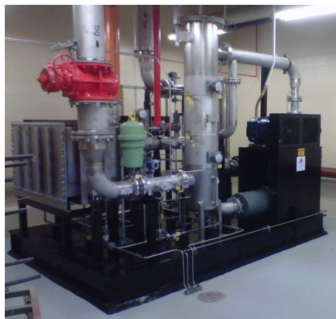
Figure 4-3 Representative Biogas Booster System
