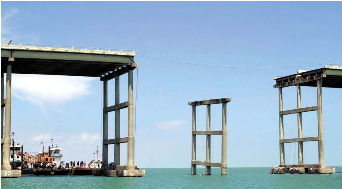
Figure 1.4 Queen Isabella Causeway collapse in Brownville, TX ( http://en.wikipedia.org/wiki/Queen_Isabella_Causeway )
