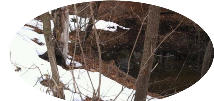
Culvert Under Rail Lines Erosion and Deterioration of Structure
