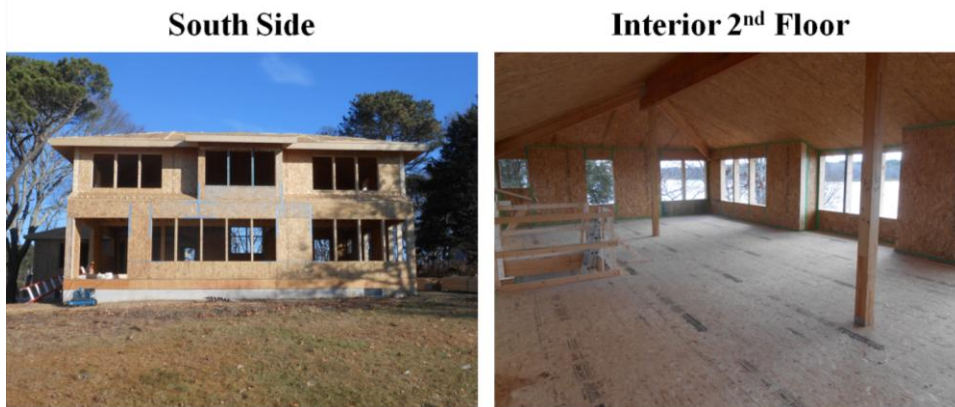
Figure 2. SIP Construction Finished. These two photos show completed panel: the exterior picture shows strapping made necessary by high winds and lots of glass. The interior picture shows the ridge beam and hips used to support the hip roof and the green Siga tape used to supplement the mastic sealing panel to wood joints.
