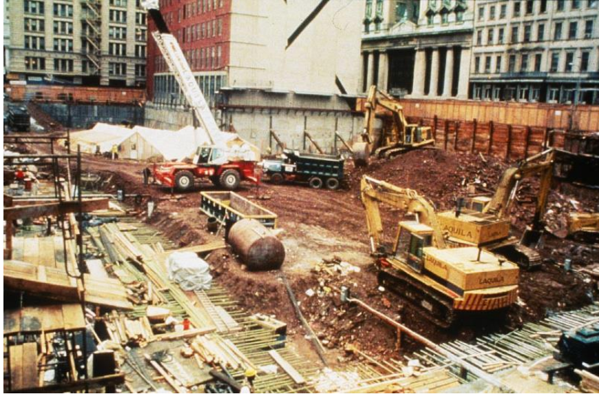
Figure 4.2: Construction and partial excavation of the African Burial Ground at the 290 Broadway Block in Lower Manhattan.
