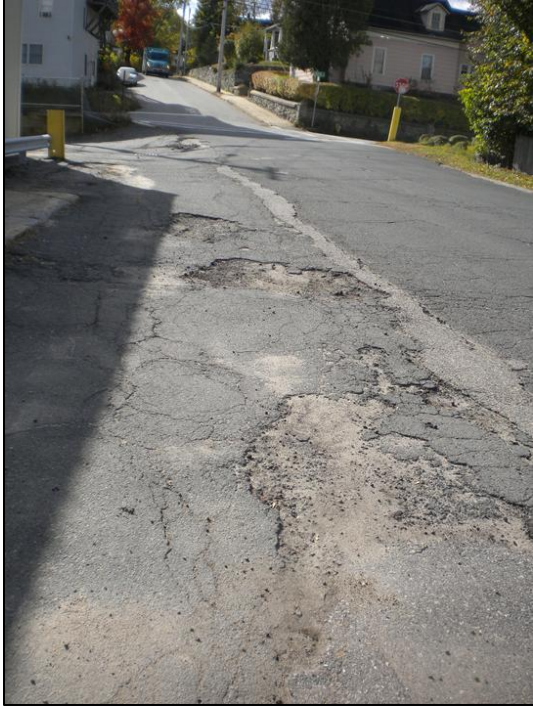
FIGURE 52: EXAMPLE OF EXISTING ROAD CONDITIONS
