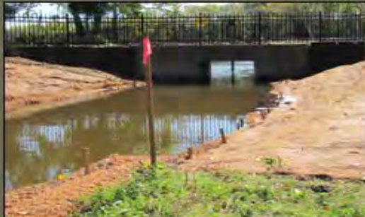
The fishway exit, providing fish access to the Milwaukee River upstream of the dam
