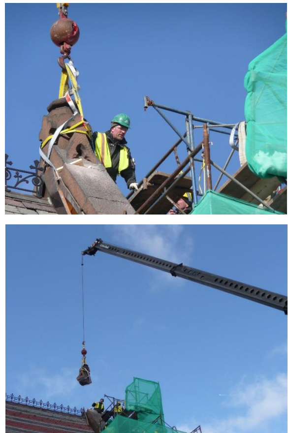
Figure 4.2. Hoisting the keystone from the east gable. On six stories of scaffolding, an Allegrone mason readies the hoisting system. Photos, the author.
