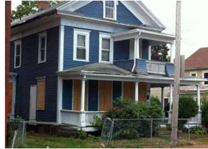
Abandoned Homes and vacant lots reflect low income and low property values
