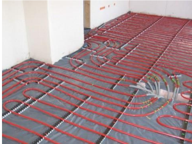
Figure 4-1. An example of the layout for a hydronic heating system. Concrete would be poured over the pipes. (Russel, 2012)
