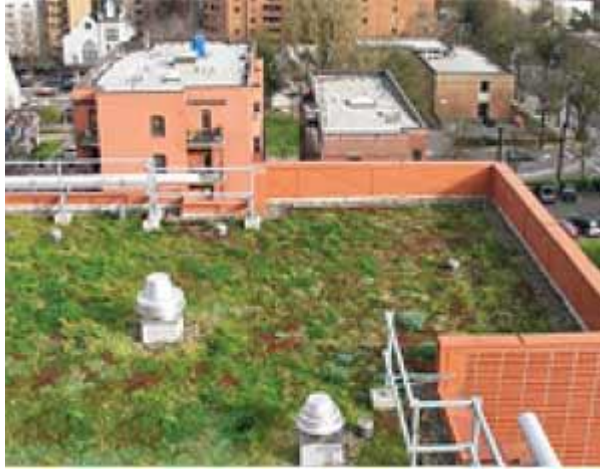
Figure 4-8. A green roof in Portland, Oregon. (Green Roofs, 2013)
