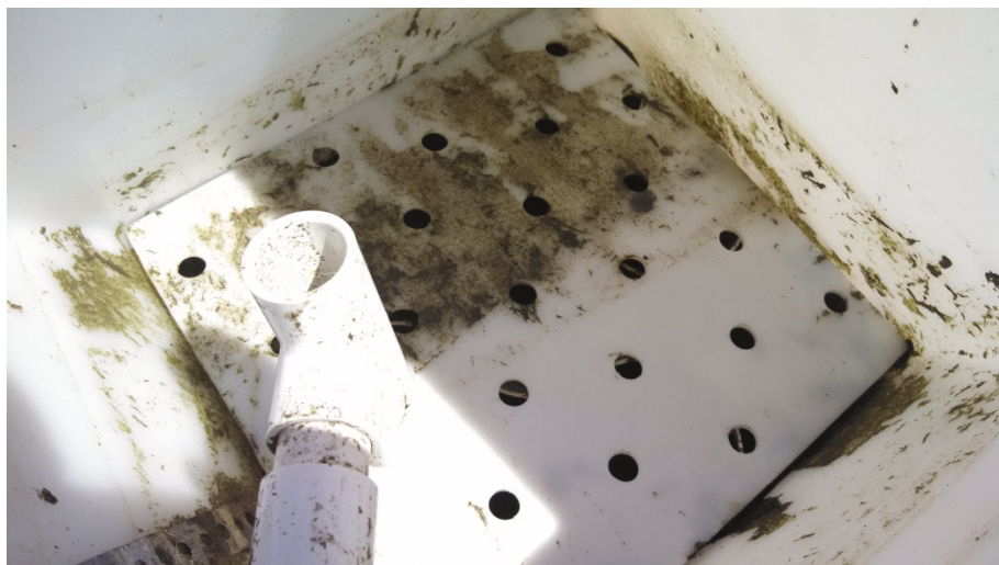
Figure 3-23: The view from the top of tube settler reveals the submerged effluent drain and the perforated backpressure plate in place. In this image, water was drained from the tube settler, while under normal operating conditions the backpressure plated is submerged in water (Chang, 2014).
