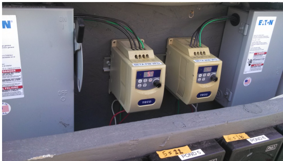
Figure 3-17: Variable frequency drives controlled the rotation speed of the water and paddle wheel motors (Chang, 2014).
