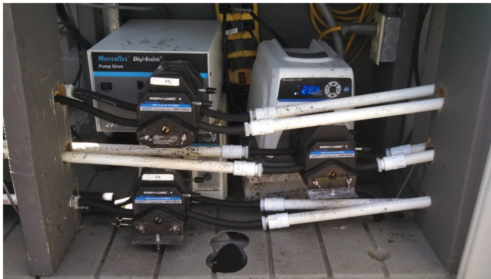
Figure 3-13: Peristaltic pumps located in the pump house in front of ponds 4, 5, and 6 to move effluent pond water from the Round-1 to the Round-2 pond sets. Each pump had two pump heads that corresponded to a specific pond and an individual tube settler (Chang, 2014).
