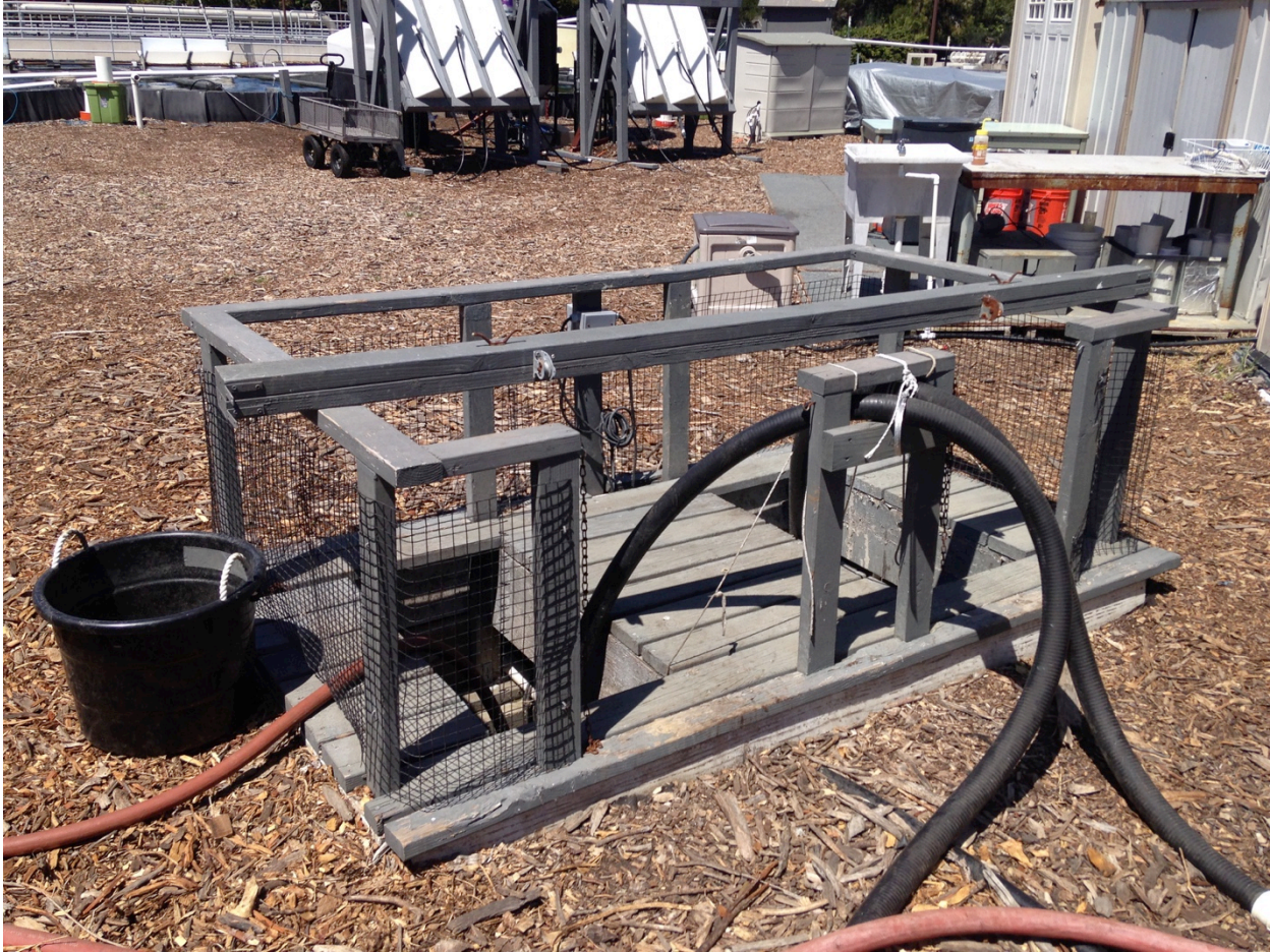
Figure 3-16: The gravity-fed AFS effluent sump had two water removal pumps that carried effluent water to the primary clarifier effluent.
