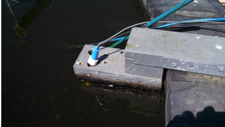
Figure 3-19: Neptune SCADA probes for DO, temperature, and pH were submerged at the edge of each raceway pond (Chang, 2014).
