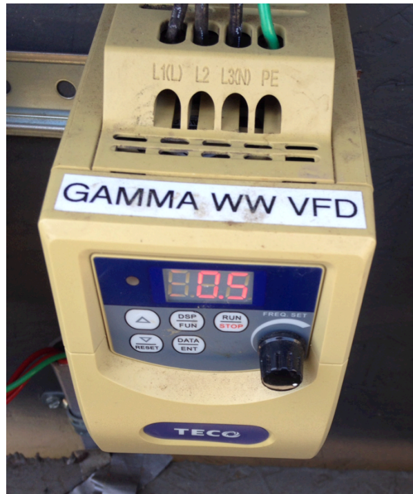
Figure 3-18: Variable frequency drive used to operate the rotational speed of the waterwheel in the 2-day HRT pond set.
