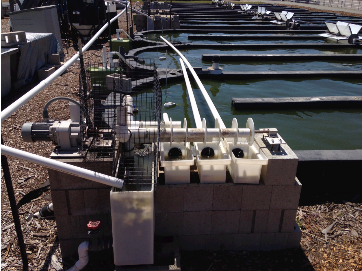
Figure 3-7: Influent waterwheel distribution system is shown feeding ponds 7, 8 and 9 at the AFS.
